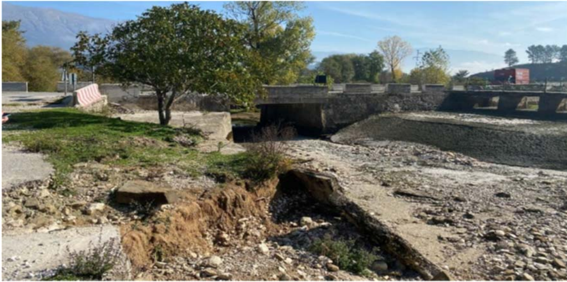
Figure 15: Damages to the structures and the lake bed after the high water levels.
