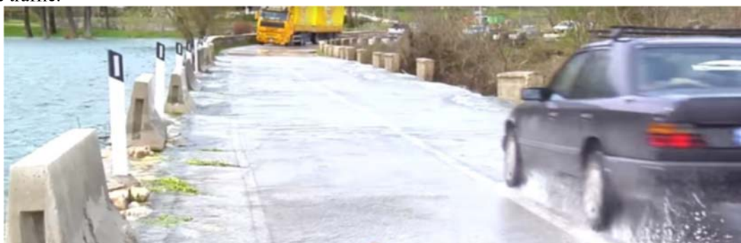
Figure 14: Lake Viroi water level over the road segment and the bridge
